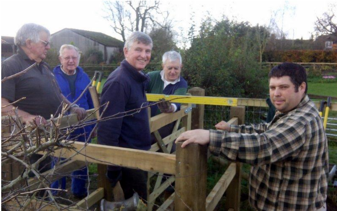
The first kissing gate nearing completion. Paul and Ken from Wiltshire Council on either side, assisted by Brian, Paul and Cedric
